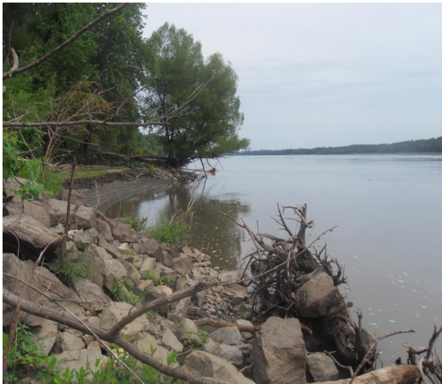
Figure 36: Bank Erosion between RM 10 and RM 9 after 2011 Flood
