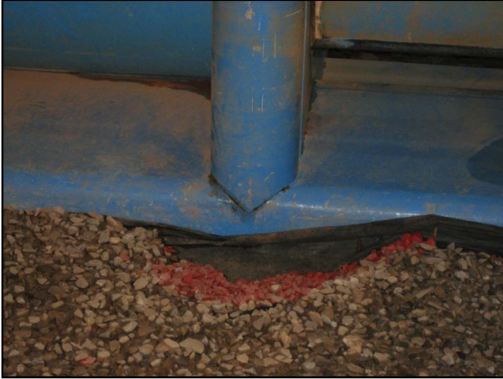
Figure 19 - Close up on right pier scour after testing with a 13 - 14 ft ice raft draft
