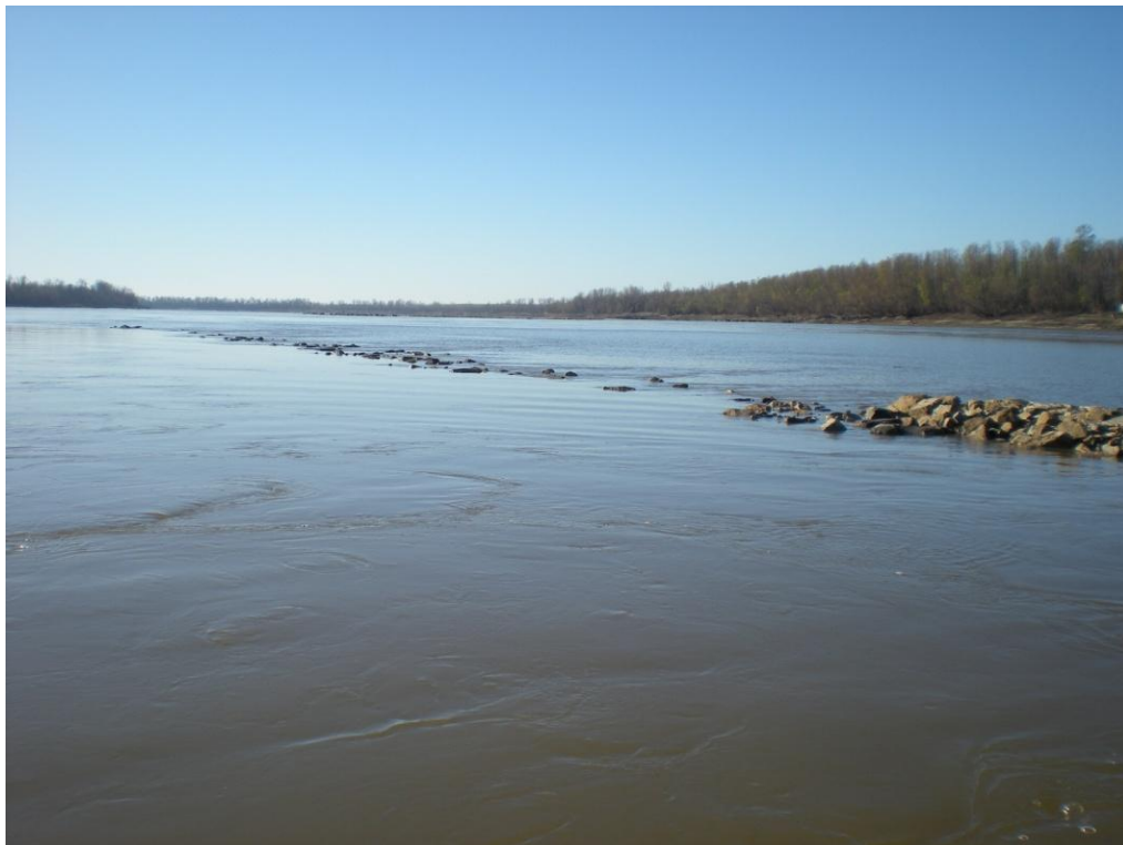
Photo 1. Navigation side leg of chevron in the Standard Chevron Field (RM 32) partially submerged. Thebes gage at 15.48 feet. November 30, 2011.
